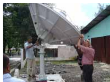
Satellite installation at the Regional Media House in Ermera. Photo: ICFJ
